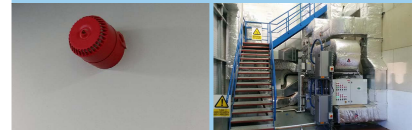
VESDA Fire Detection System
