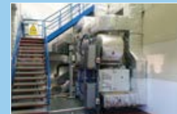
Air Conditioning Unit
