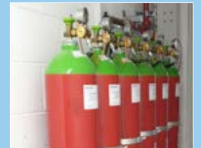
INERGEN IG541 Cylinders
